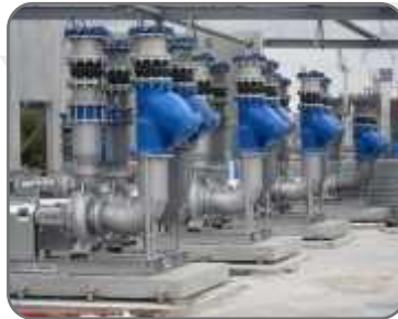
WATER PIPING SYSTEM
