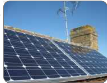
SOLAR ENERGY SYSTEM
